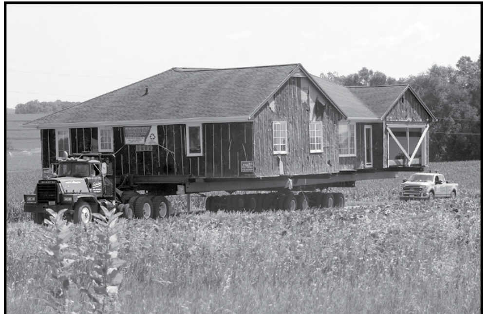
Work was done on the former WSC Alumni House before it was moved to its new location.
