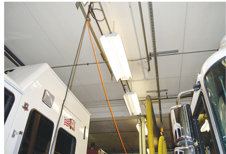
Ceiling is too low
