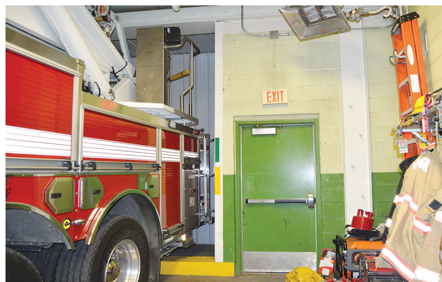
Part of the back wall was blown out to have room for the trucks
