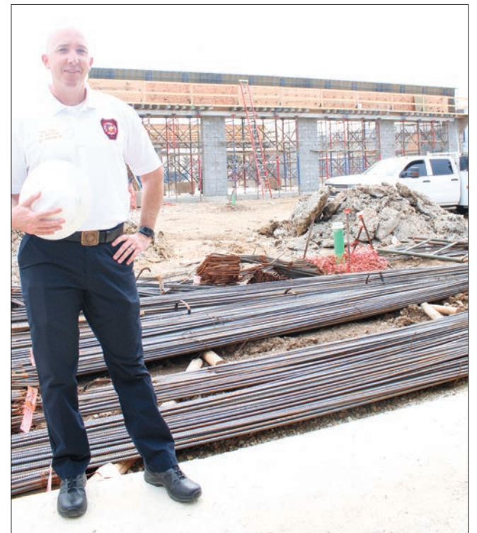
JOLEE SKINNER | TRI-COUNTY REPORTER Lake Worth Fire Chief Ryan Arthur is standing on site of a new fire station currently being constructed.
