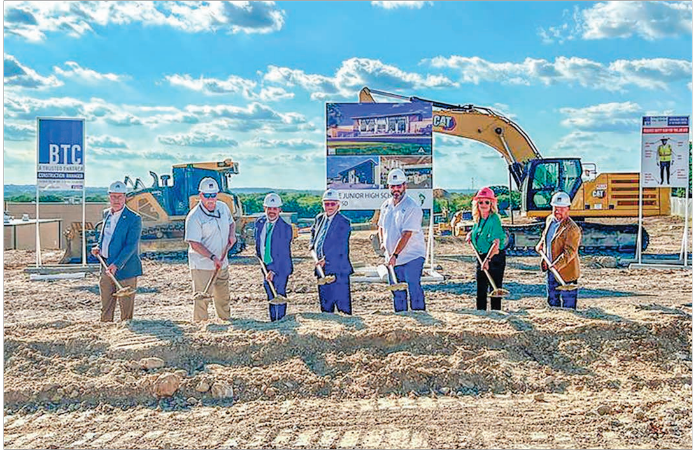
Azle ISD trustees get to work moving dirt at the construction site.
