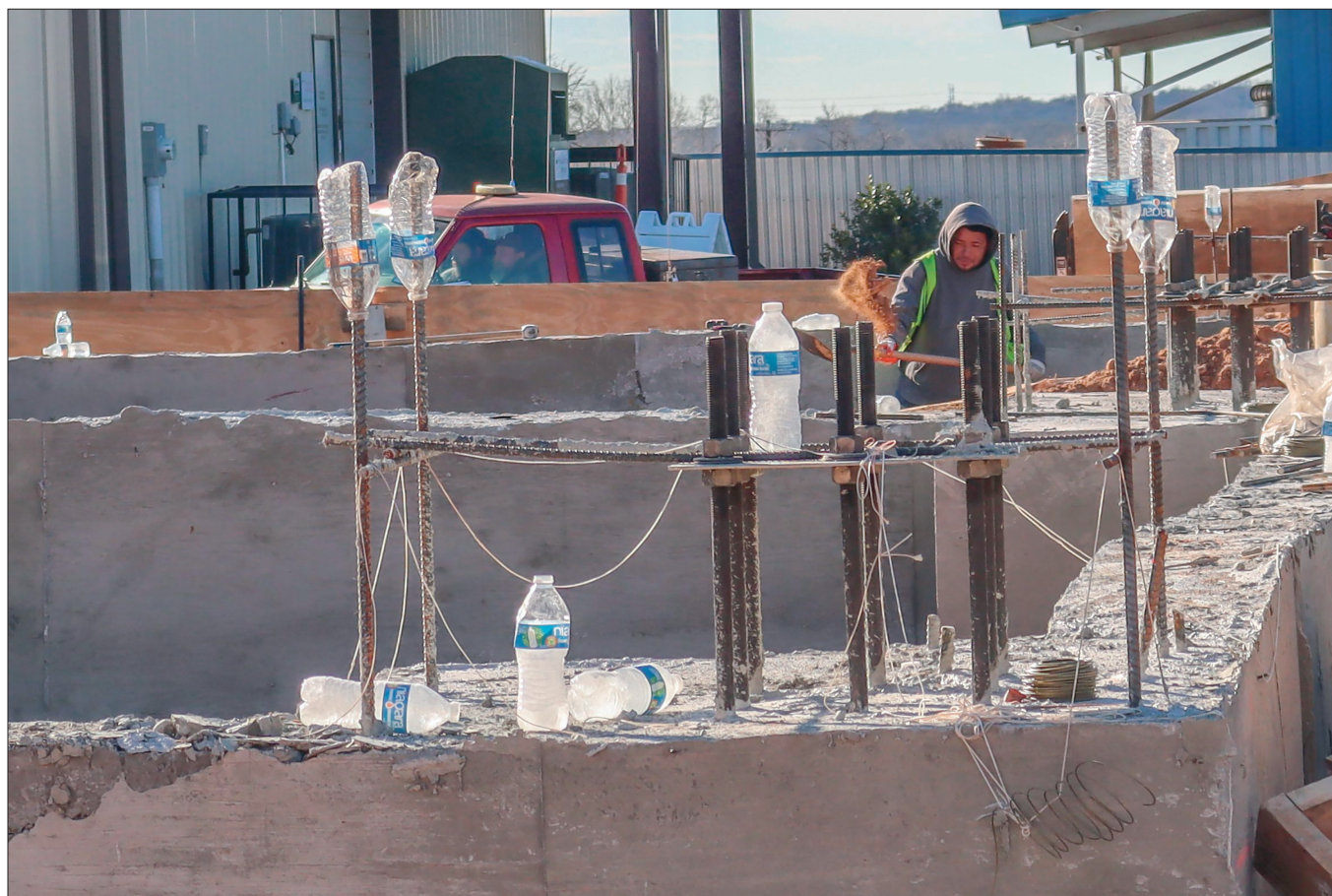
Water bottles cap the rebar at the recently started site of the expansion.
