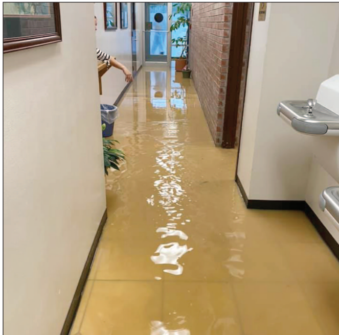
Water coming into the Parker County Sheriff's Office building in Weatherford during heavy rainfall May 24.
