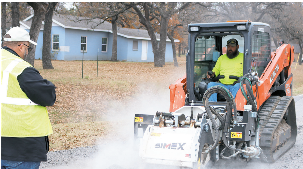
Azle streets employee Jeremiah Johnson uses a skid steer with milling machine attachment on a repair job on Ash Avenue near Park Street, as streets superintendent James Duvall looks on. A hot mix (asphalt) was used on the street. Photo by Don Munsch
