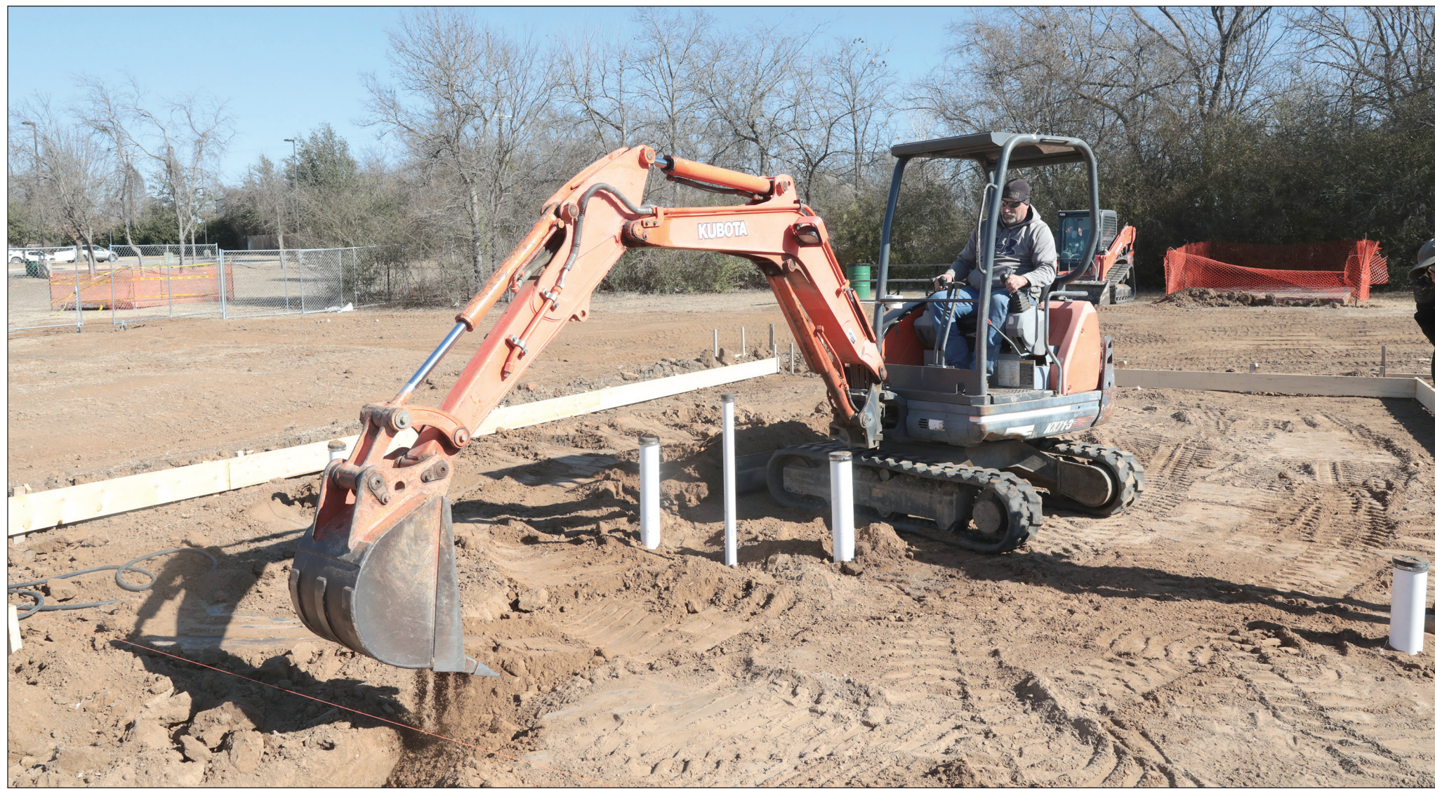
Crews, including Larry James on Tuesday, started work in January on the site of the new restroom building and splash pad at Central Park in Azle.
