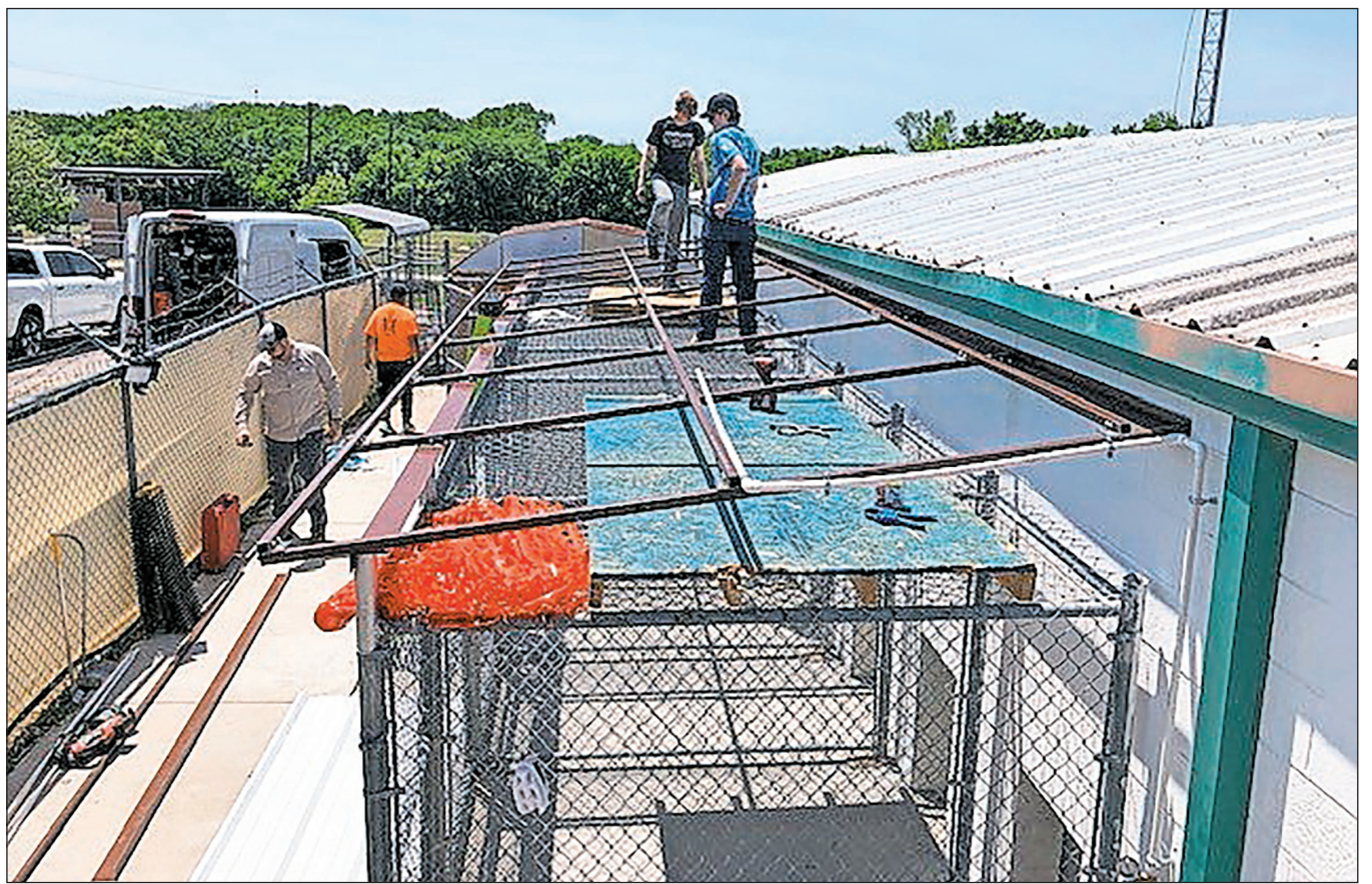
Troop 175 was able to replace the roofing, rewelding some of the points, and also installed a misting system.
