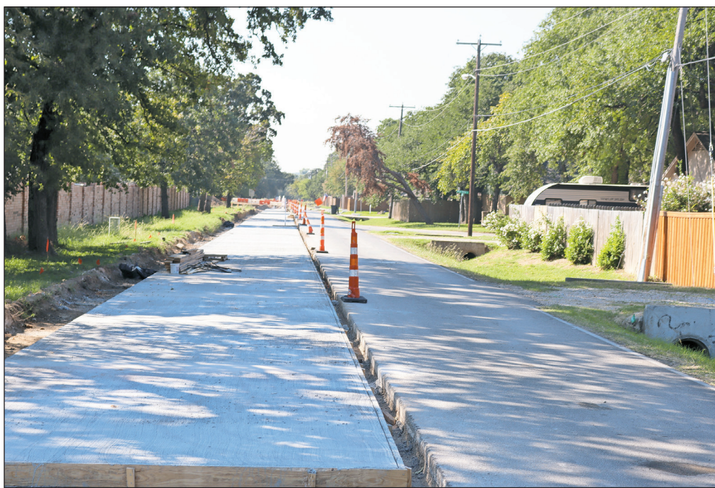
PHOTO BY DON MUNSCH Concrete has begun to be poured on portions of Ash Street. This portion is near Lake Ridge Drive.
