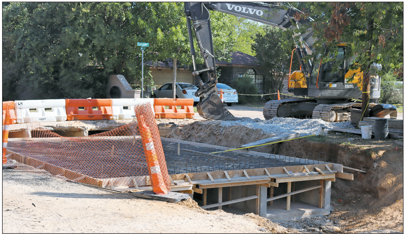
PHOTO BY DON MUNSCH Box culverts are being created along Ash Street.
