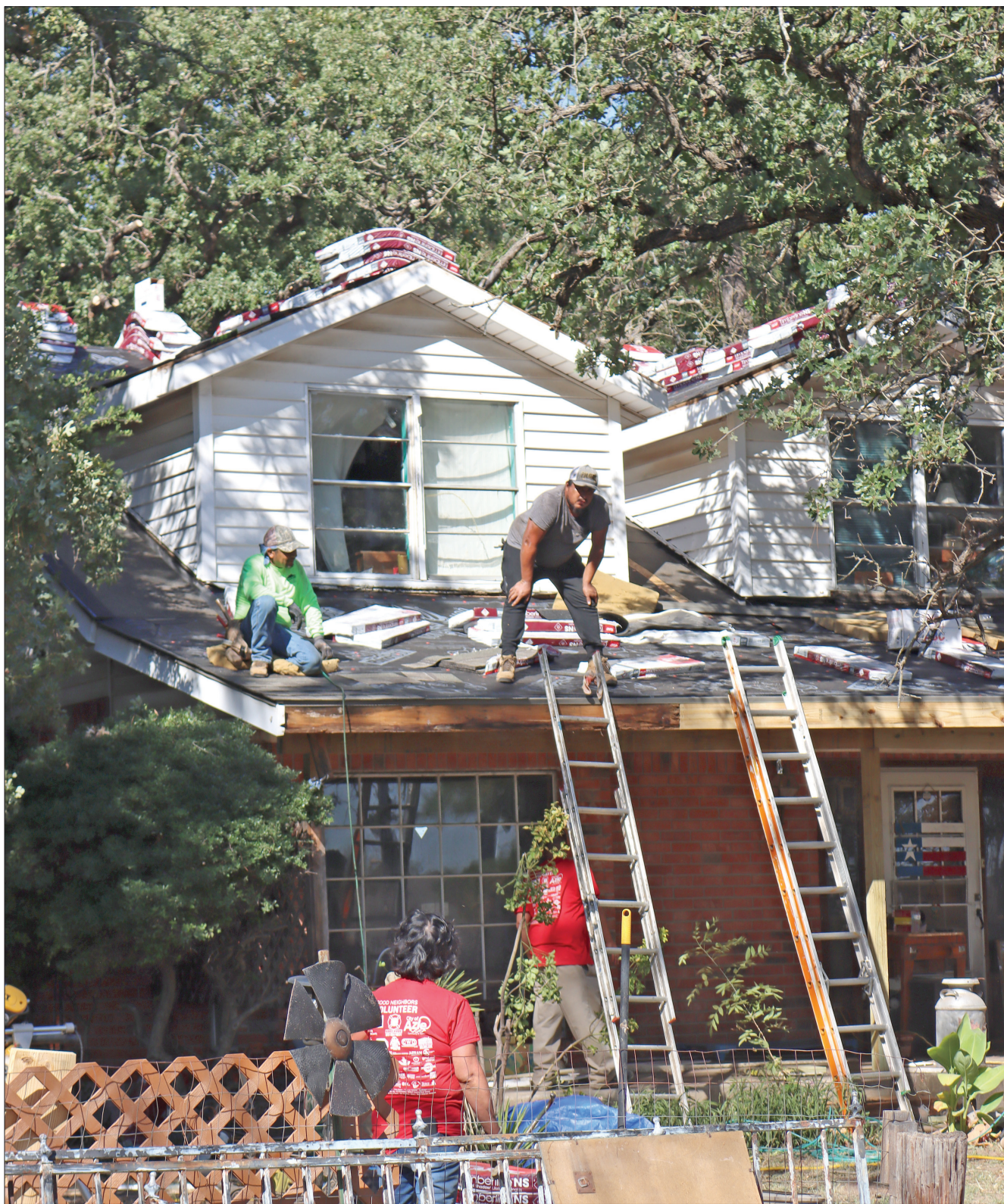
PHOTO BY DON MUNSCH A home renovated during the Good Neighbor Blitz gets a new roof.
