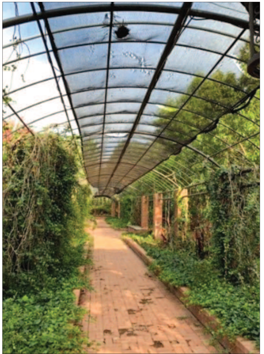
COURTESY PHOTO The brick arbor at Clark Gardens was damaged during Winter Storm Uri 2021, causing many bricks to crumble to dust.
