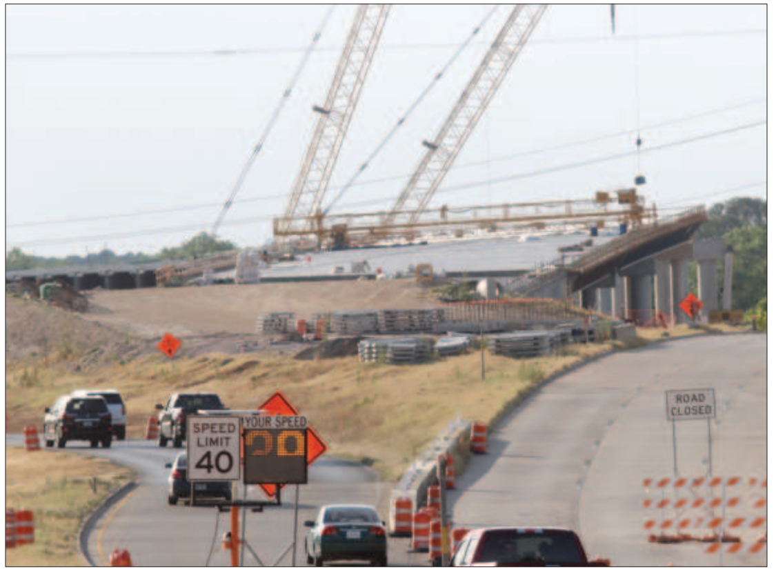
PHOTO BY DON MUNSCHE Northbound on SH199 at the Lake Worth bridge. The bridge project is still two years from completion.
