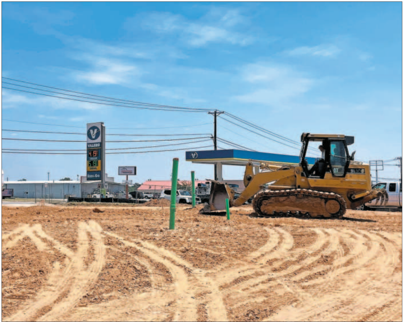
Melville’s work has started at the Jack in the Box location in Springtown.
