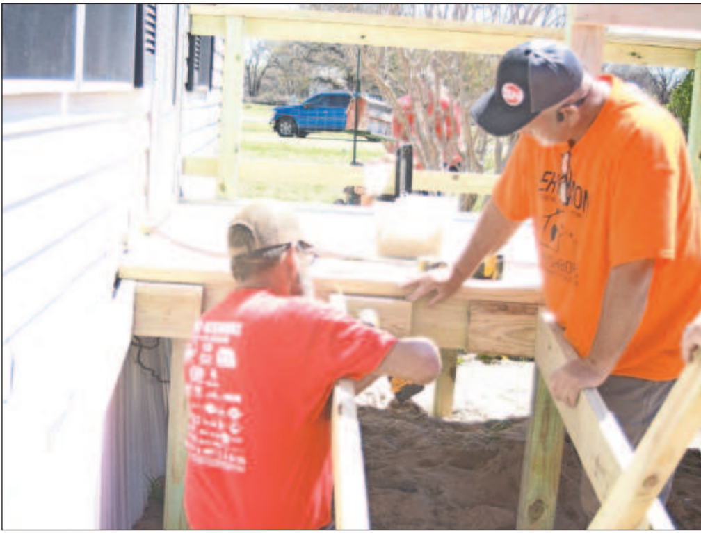
Gary Dart and Robby Kent of Dynamic Decks helped build decks with Servolution at the Spring Blitz on April 8-9.
