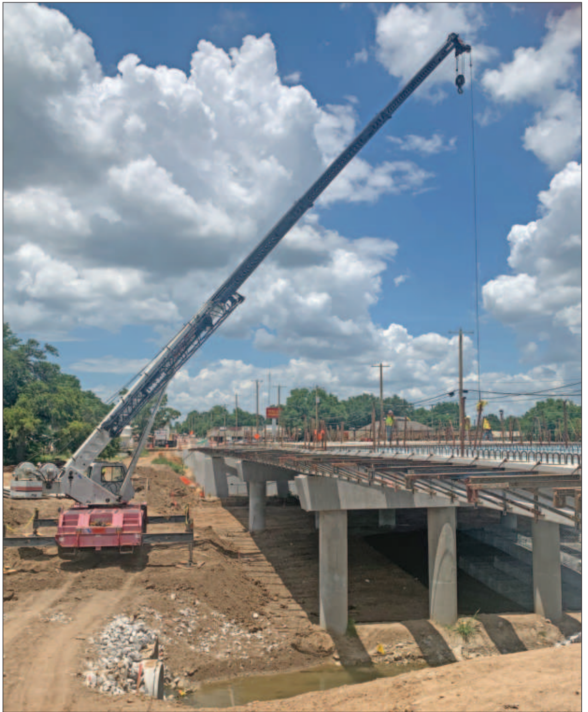
Bridge beams were recently installed and preparations for the bridge deck are ongoing.
