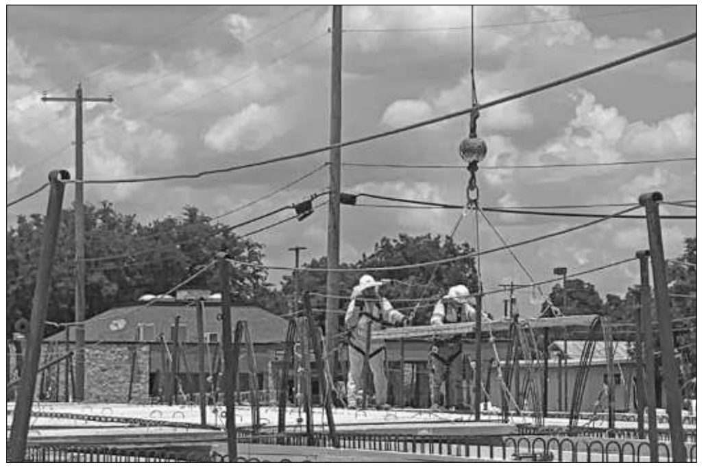
The improvements to FM 51, the bridge, and Hwy. 199 will allow for better traffic flow, pedestrian access, and will bring the bridge and the intersection of the two roadways out of the 100-year floodplain. Photo by Kim Ware
