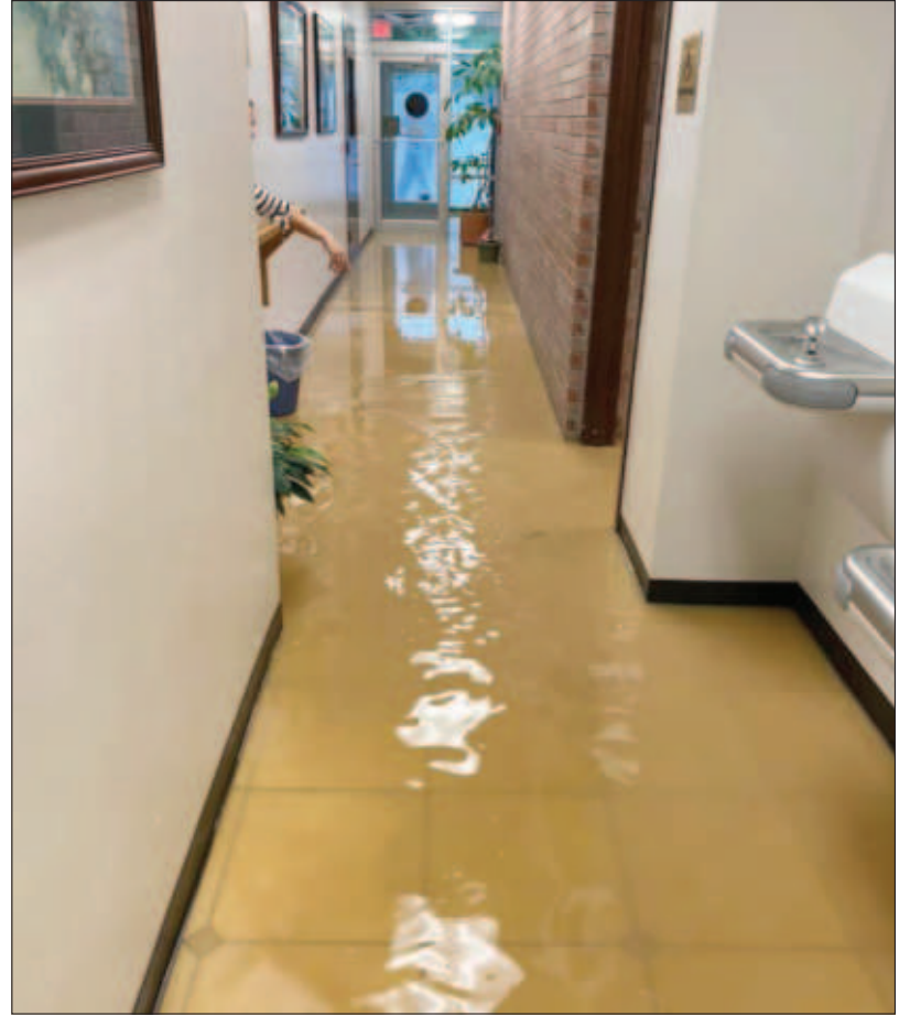
Water coming into the Parker County Sheriff's Office building in Weatherford during heavy rainfall May 24. Photo courtesy Parker County Sheriff's Office
