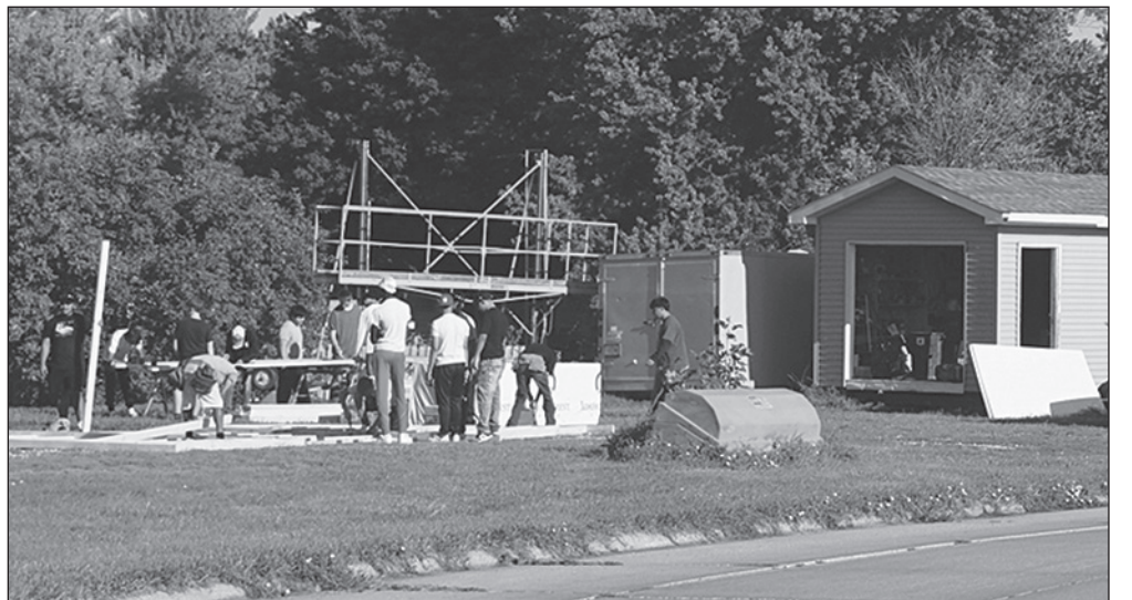
The heat isn't slowing down the Storm Lake High School Building Trades class as they spend their morning hard at work in their outdoor classroom.
