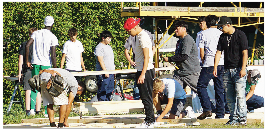
The heat isn't slowing down the Storm Lake High School Building Trades class as they spend their morning hard at work in their outdoor classroom.
