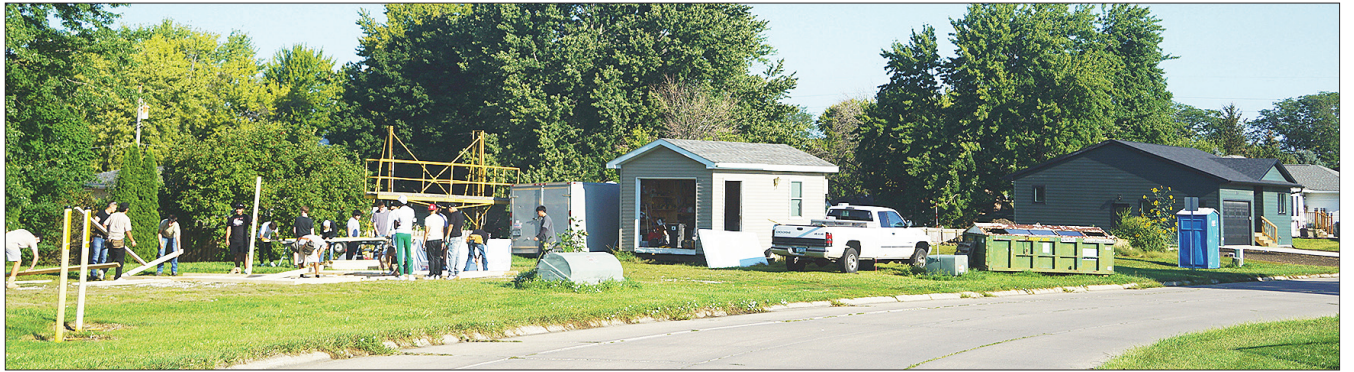
The Storm Lake High School Building Trades class is hard at work on the latest project just a lot away from the program's most recently completed project.
