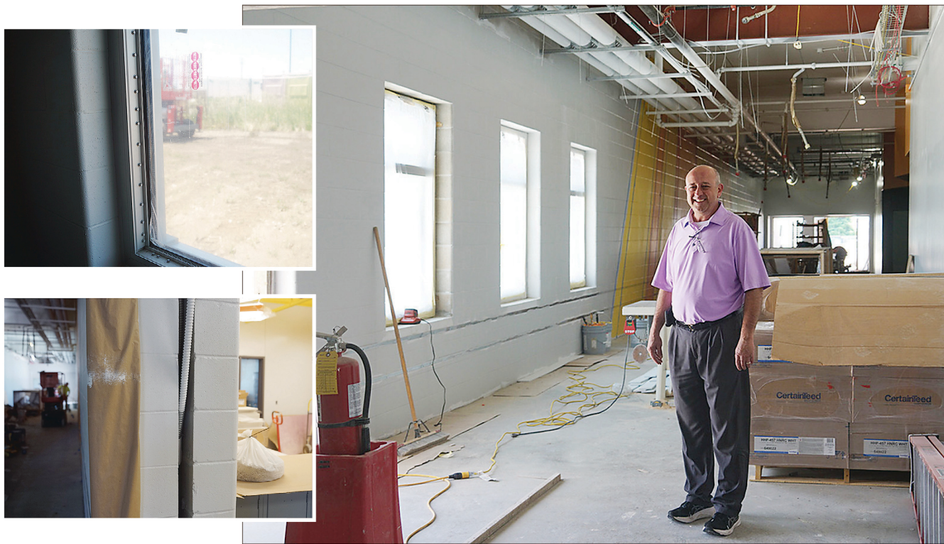
Storm Lake CSD Jeff Tollefson shows off the area in the new wing at the Early Elementary building that will not only hold first grade classrooms but will also double as a tornado shelter. Above left: The windows in the shelter are extra reinforced. They can withstand an impact up to a hundred miles per hour. Left: The walls feature double bricks and cement along with extra reinforcements in between.
