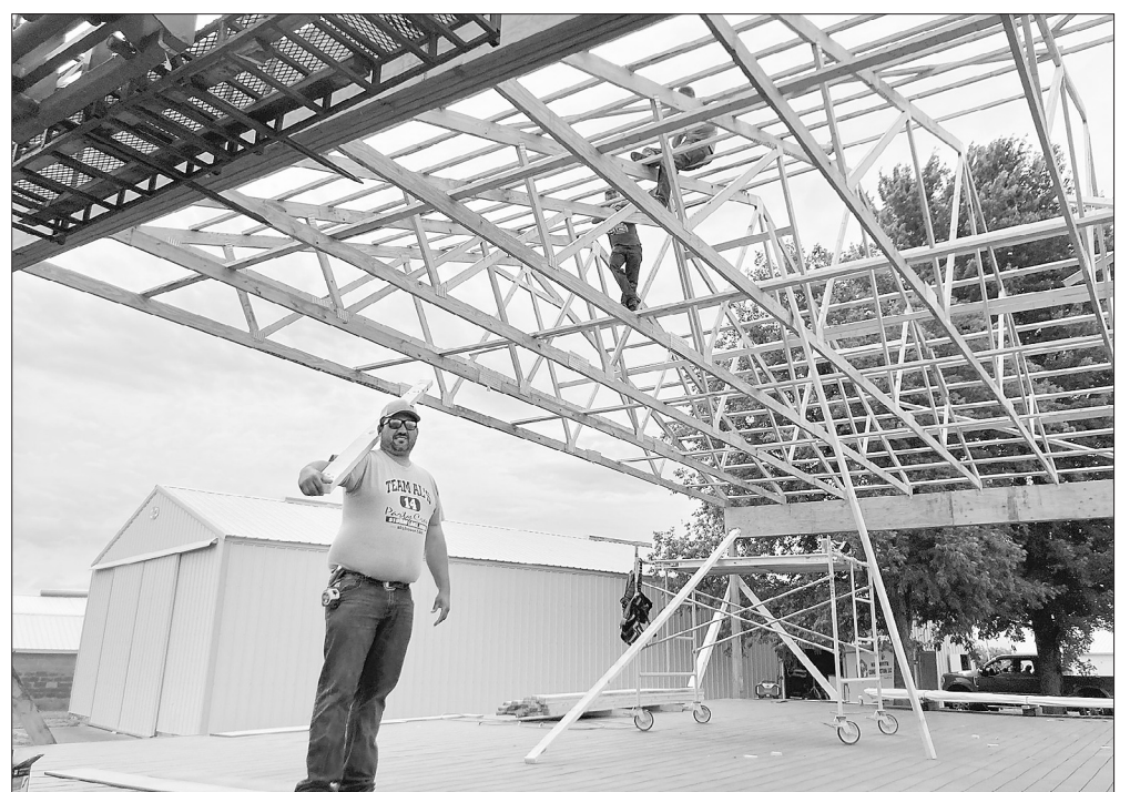
At work Wednesday on the new roof for the stage are, up front, Mike Christen, and above, Dylan Reimers and J.J. Phillips. Also helping on the project are Dean Phillips and Justin Hocking. The 32' x 50' stage was in place last year, but it had no covering. TIMES PILOT photo by DOLORES CULLEN
