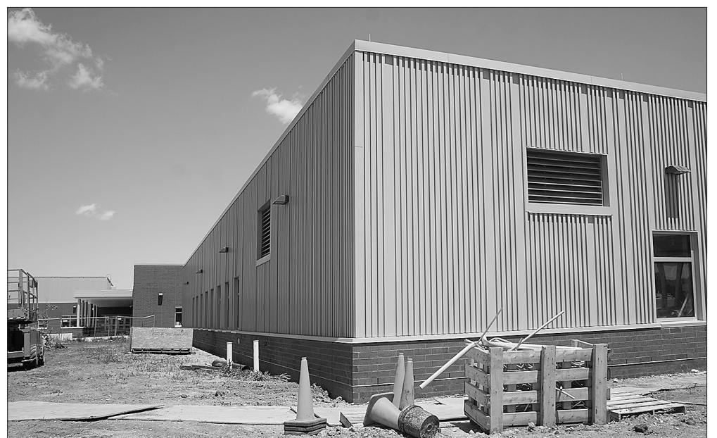
The tornado shelter at the Early Elementary School features external reinforcements as well as a roof that includes several inches of brick as well as several inches of cement making it a rated tornado shelter. The main entrance of the building can be seen at far left.
