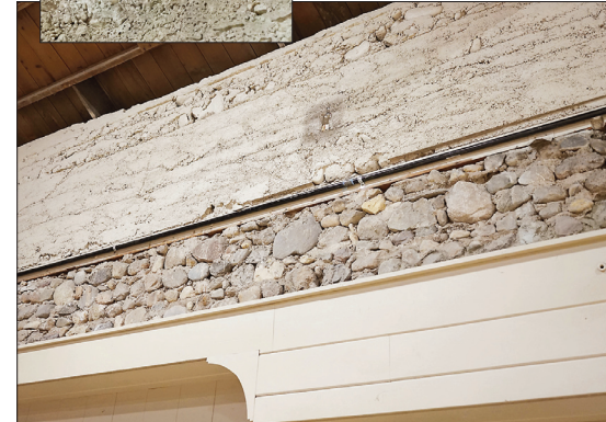
A mysterious liquor bottle, left, is embedded in the masonry of a wall in the ballroom. Can you see it below in the upper center part of the photo?
