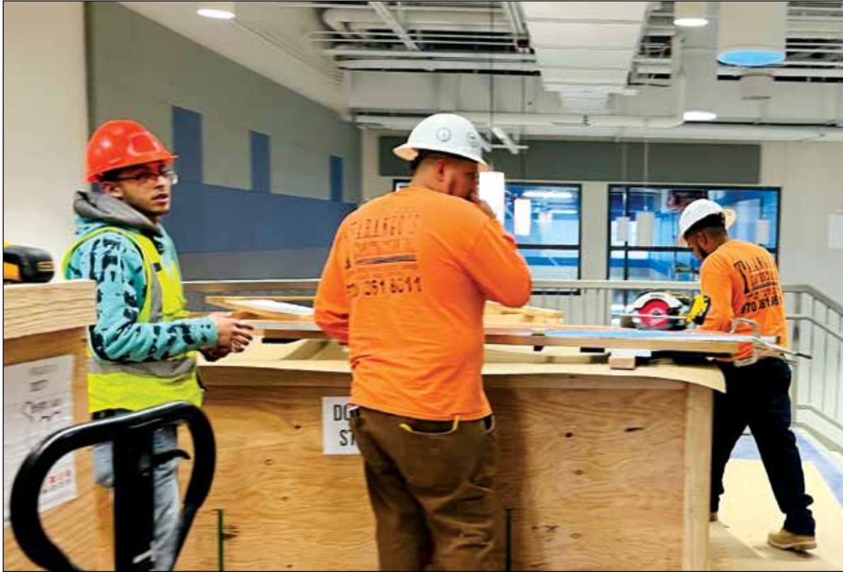
Contractors execute the finishing touches of the ceiling in the entryway of the new school on Dec. 29.
