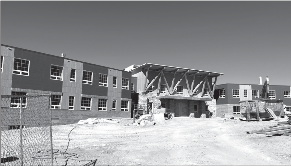
The new K-12 in Nucla is still on schedule to be completed around the holidays. (Photo by Regan Tuttle)
