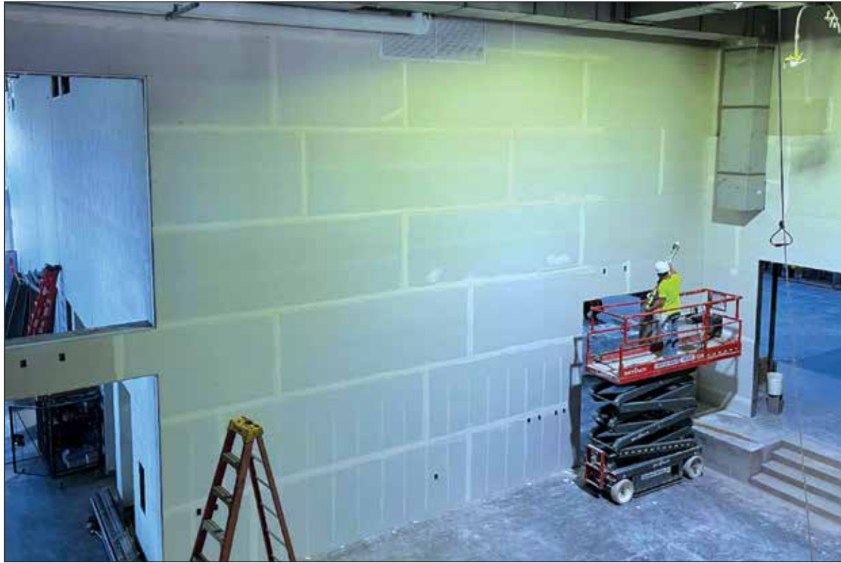
FCI crews finish drywall on the lower level of the new school. (Photo by Clint Wytulka)
