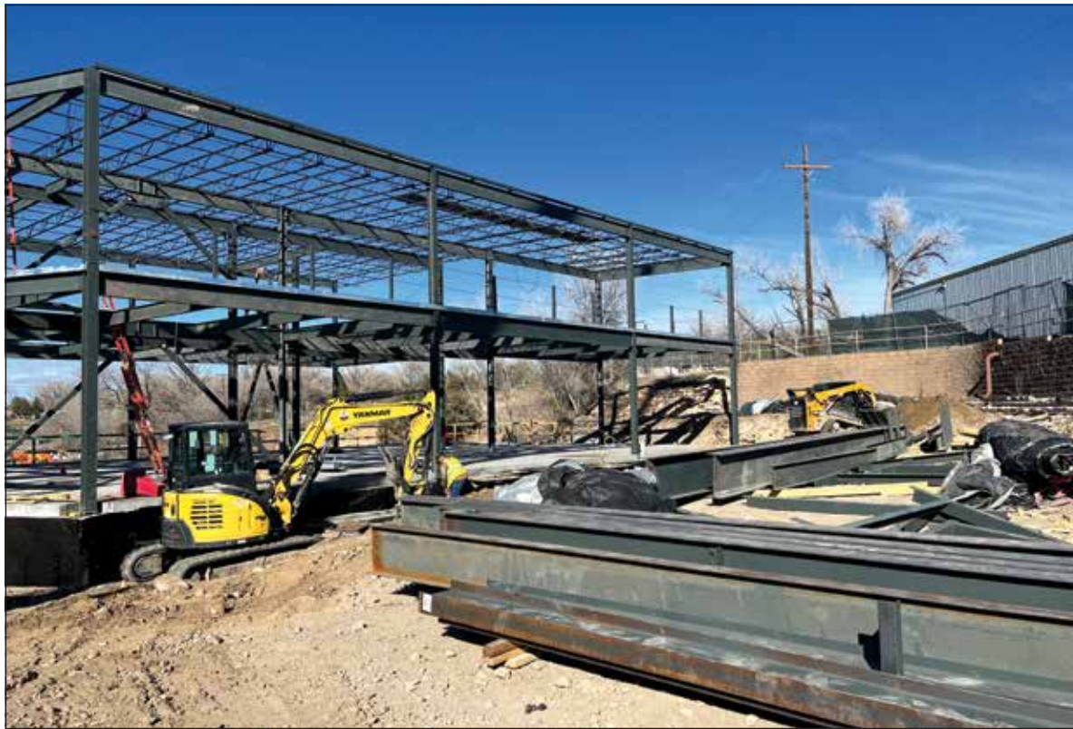
The new school in Nucla receives another $750,000 from the state's Department of Local Affairs. (Photo by Regan Tuttle)
