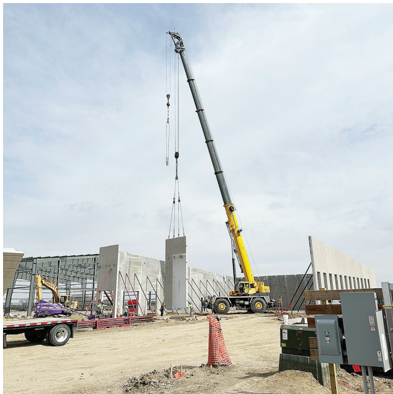
PHOTO COURTESY CITY OF SEWARD
