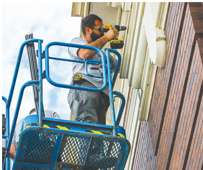
FILE PHOTO City of Seward workers install lights on the city hall building in 2022.
