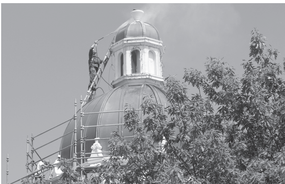
Lindner Painting crews last week water blasted the domes of the Seward County Courthouse. Priming and painting of the dome and structure are expected to begin soon.
