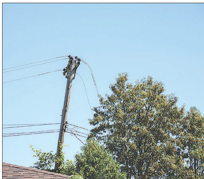
You are not imagining things and it is not an optical illusion, the pole is leaning due to the damage caused by the trees that fell on the wires. Several poles in the line could be seen leaning severely and, in this case, the broken lines are also visible. Photo by Bruce Karnick
