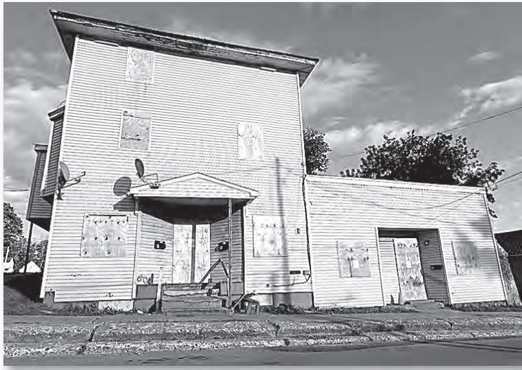
Village of Massena Code Enforcement officers have shuttered the property located at 18 Park Avenue following a failed fire inspection. The property, called a "nuisance" by many residents at a recent meeting, has been a controversy in the village for several months
