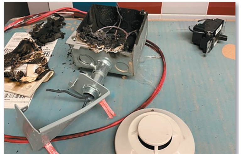
Above is what's left of an electrical box that caught fire at the school.
