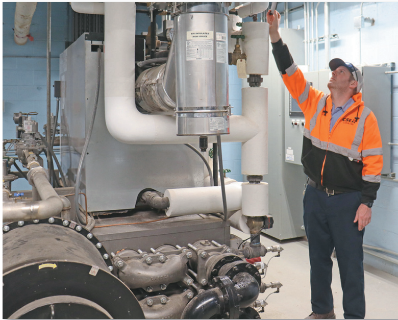
Village employee Justin McGrath regulates the dual-fuel boiler used to heat the digester sludge at the Potsdam Wastewater Treatment Plant.
