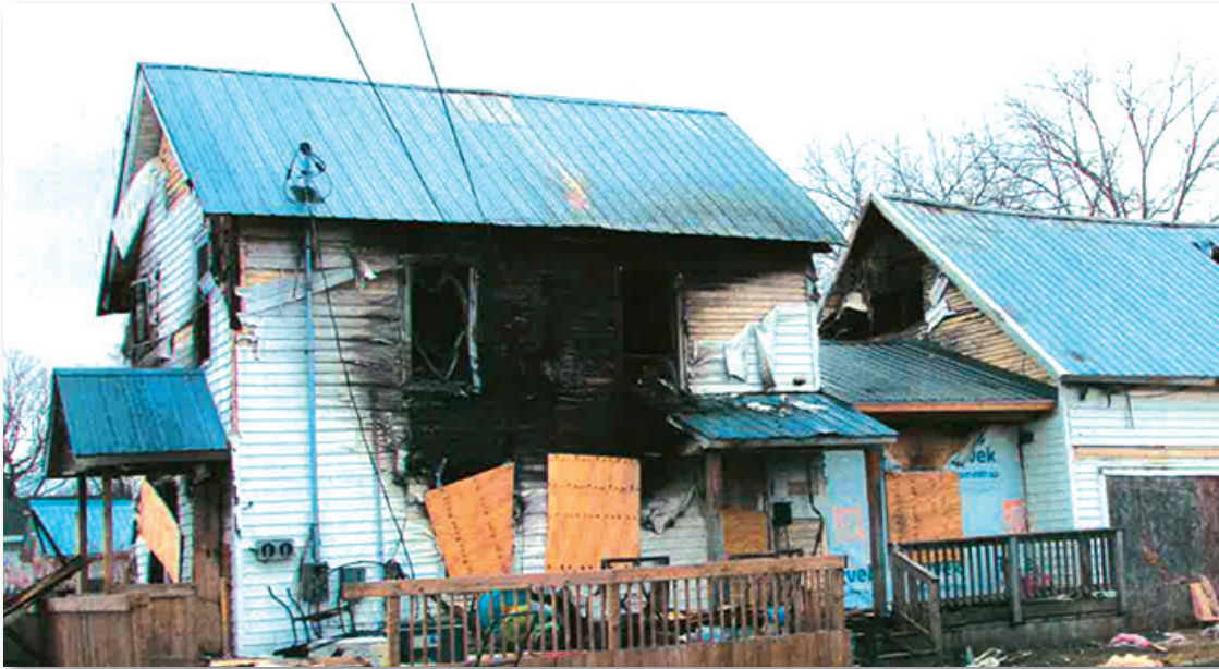
Village of Massena officials are moving forward with plans to remove a blighted property at 23 1/2 East Orvis Street, which was damaged by fire in April 2022. Trustees formally approved demolition in Sept. 2023.
