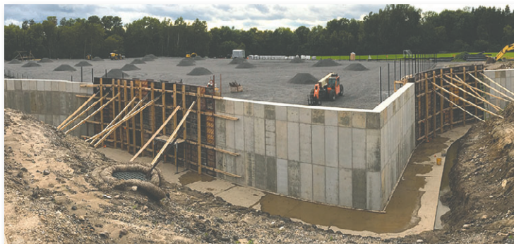
Construction on several aspects of Canton Central School’s capital project will continue throughout the school year.
