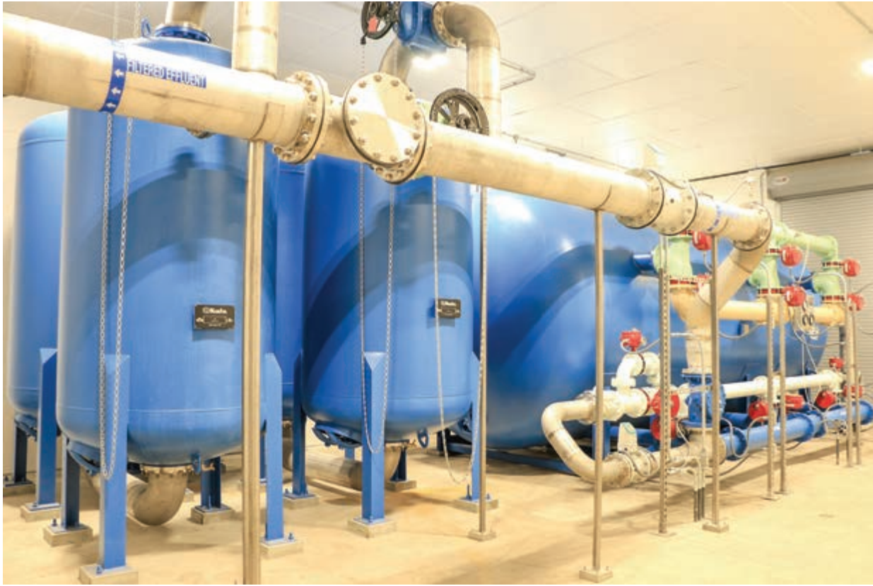
Kronenwetter's new filtration system is expected to improve water quality in the village.
