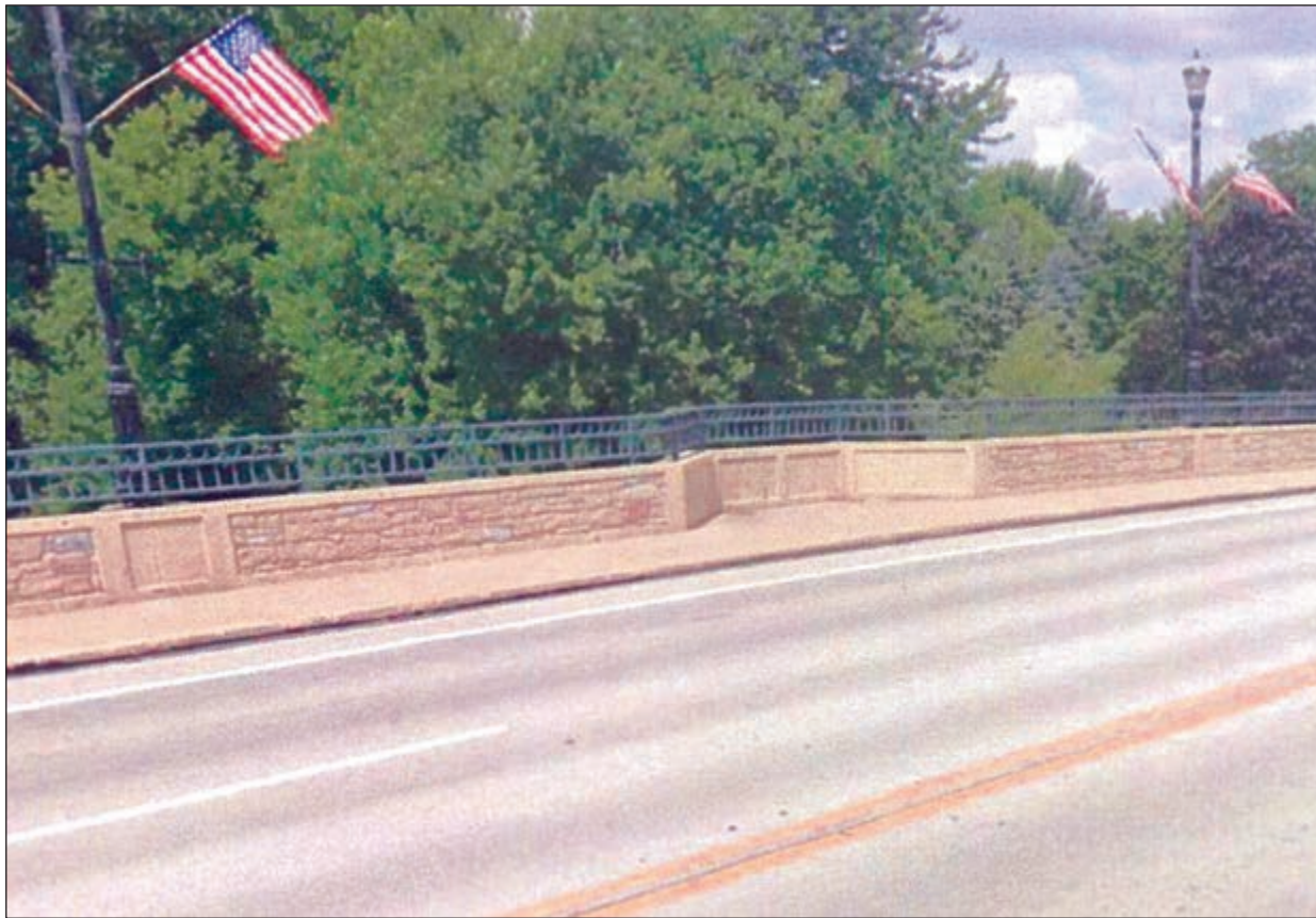
The bridge across the Fox will include a pedestrian sidewalk and six pedestrian bump outs for viewing, three on each side.
