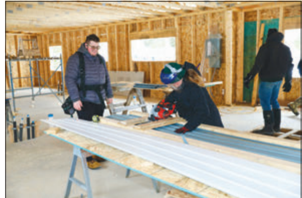
Students learn trade skills while building a home for a family in need.
