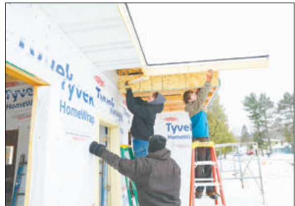
The class works daily to build a house on Coolidge Avenue, next to the high school.
