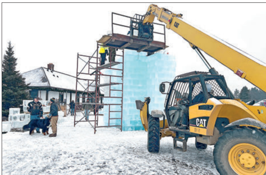
The Eagle River Fire Department used heavy equipment and scaffolding to construct the ice castle towers Friday afternoon.
