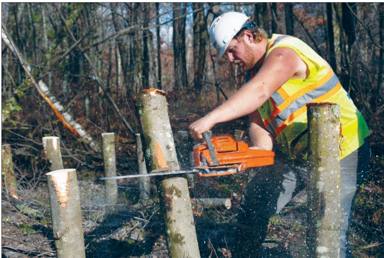
Joel Pennycamp, an employee at Hoffman Construction, cuts a log with a chainsaw while building a series of artificial beaver dams on a wooded property his boss, Jim Hoffman, owns. Joe Timmerman / Wisconsin Watch photos
