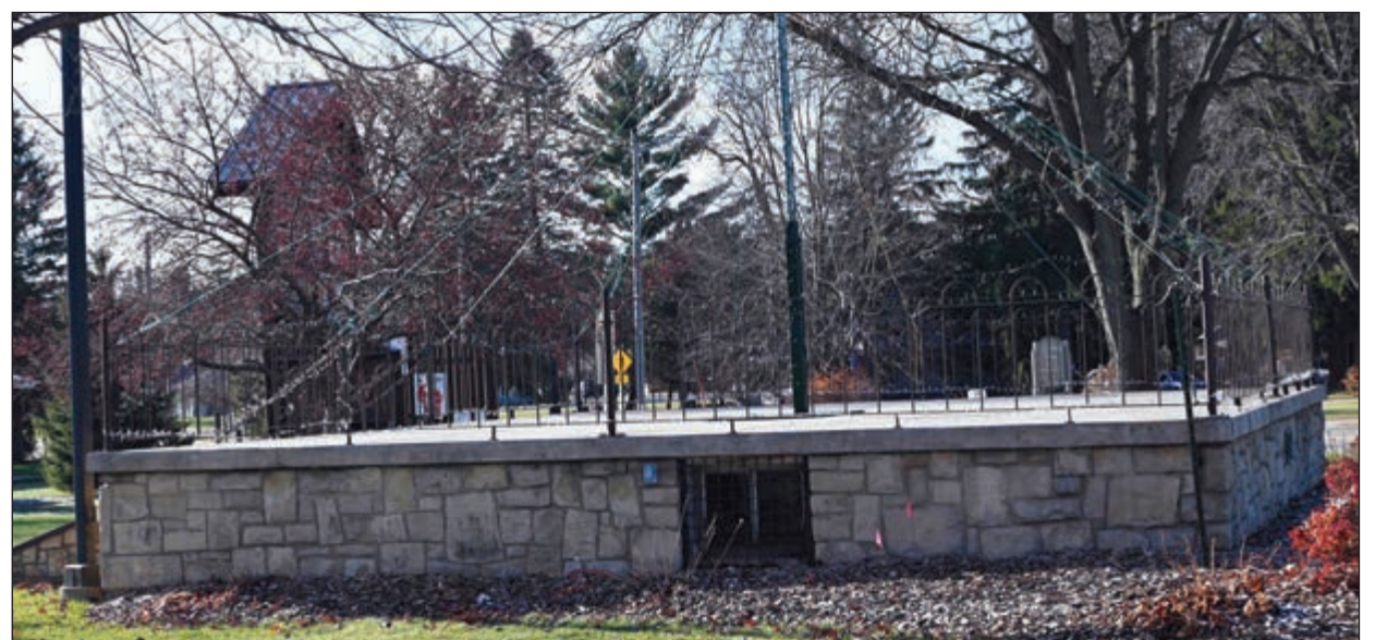
The Triangle Park Committee is looking to continue to improve the park. One of the projects includes putting a roof over the band stand along with an ADA accessible ramp.
