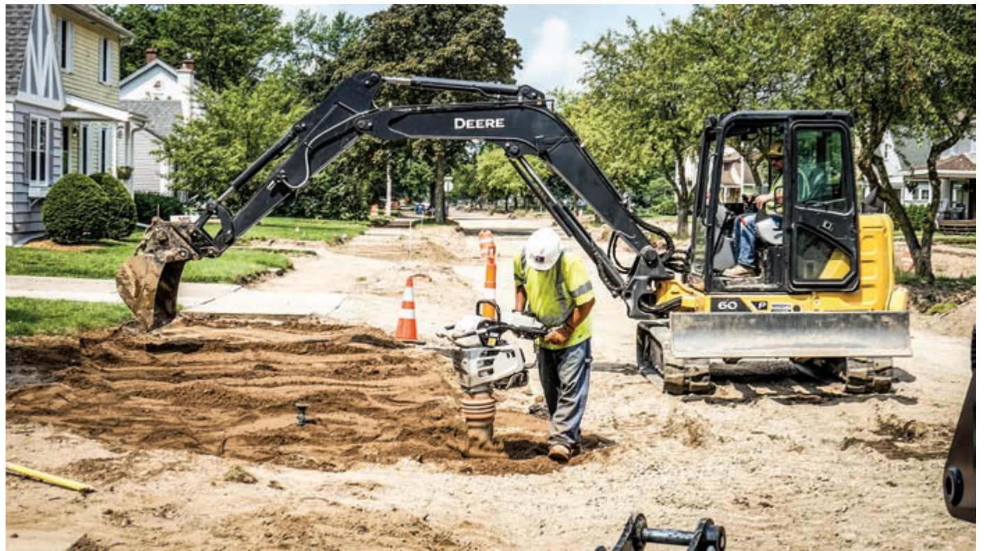
A worker smooths out dirt in front of a home on Eau Claire Boulevard after a lead pipe was replaced.
