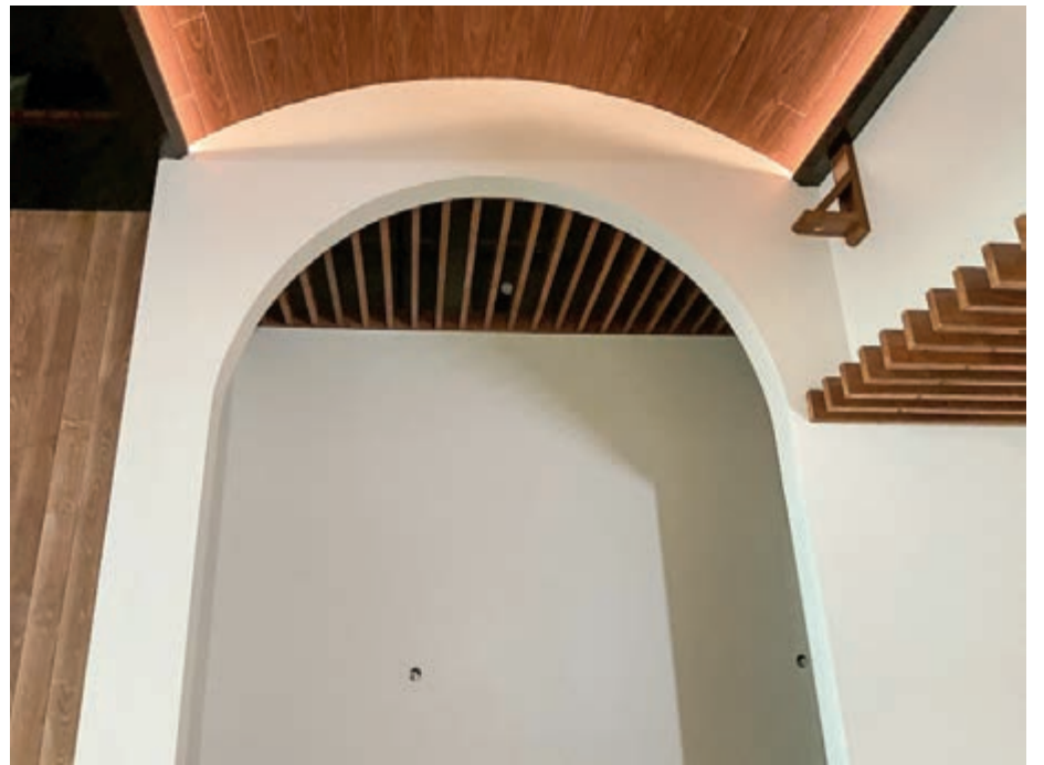
A photo submitted to the city shows some of the progress at Infused. Its developers say the project will be ready by November.
