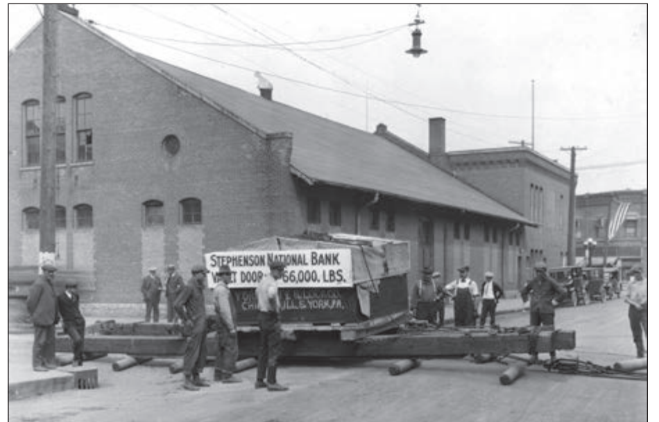
Workers roll the bank's 66,000 lb vault door across logs to the bank's front door for installation. Submitted photo
