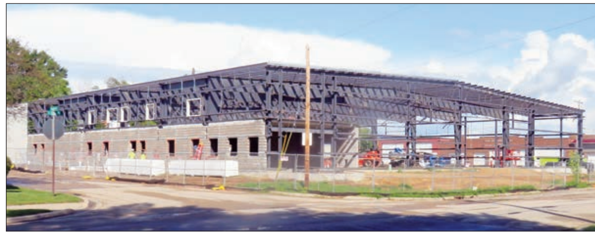
The new building being constructed for Clintonville Utilities is on schedule, and estimated to be completed around April of next year. Bert Lehman Photo
