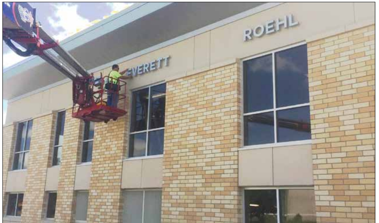
Trent Nolan with Creative Sign Company Inc. from De Pere installs the letter "e" on the Everett Roehl Marshfield Public Library on July 12, 2016. HCT Staff photo
