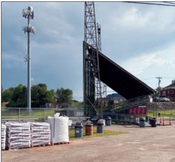
Work was halted at the stadium grandstand in Clintonville. Bert Lehman Photo
