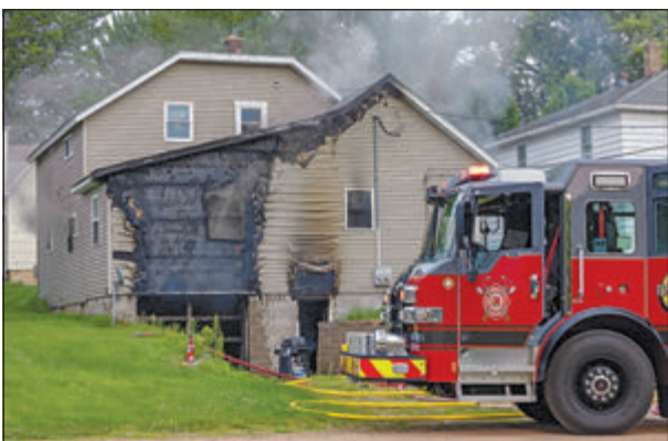
Fire departments were on scene and extinguished the blaze quickly, but not before extensive damage to both apartments in the house. Joseph Frederick photo.
