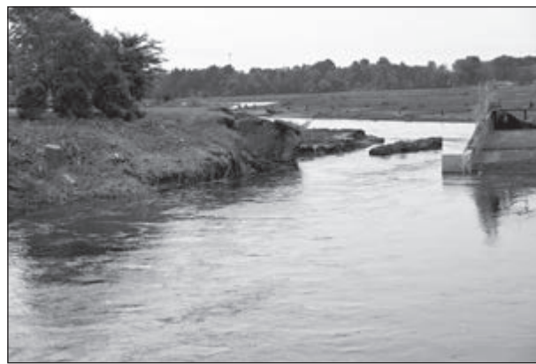
The Manawa City Council voted that they would like to rebuild the dam July 22 as the work to plan and evaluate the dam conditions continues.
