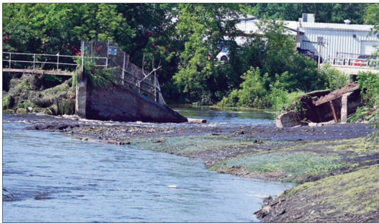
A storm on Friday, July 5, caused the dam at the Manawa Mill Pond to breach and flooding to occur in the city of Manawa. Emily Conroy Photo
