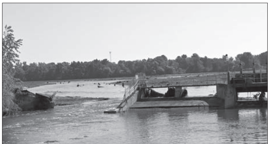
The Manawa dam was breached Friday, July 5, during a storm that brought a torrential rainfall of more than 5 inches within a few hours. Homes downstream of the dam were evacuated as streets were flooded.
