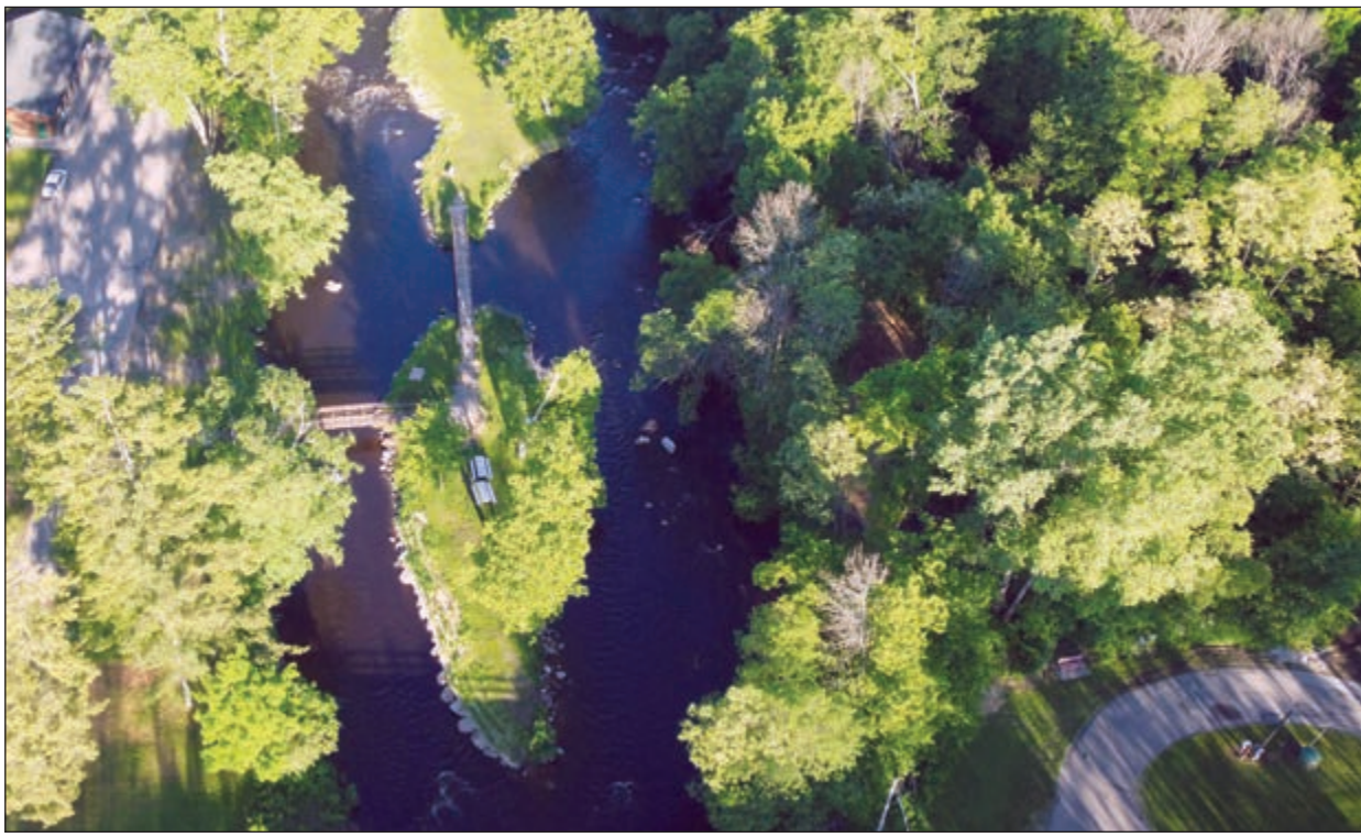
The island restoration work at Brainards Bridge Park is completed after a season of earth, rock and tree moving. Erosion was slowly washing away the islands. Wildflowers and tree were planted and dead ash trees were removed. Submitted Photo
