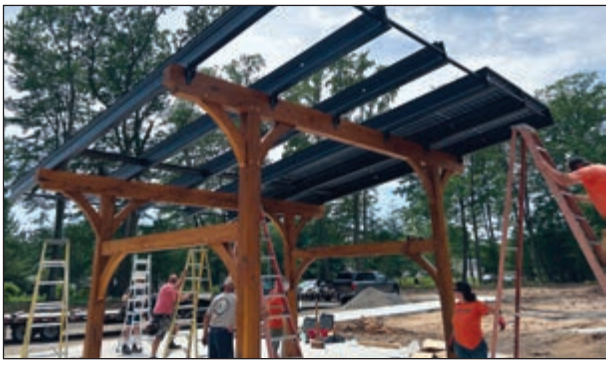
Construction crews are building a solar canopy shelter at Groholski Park in Stevens Point.
